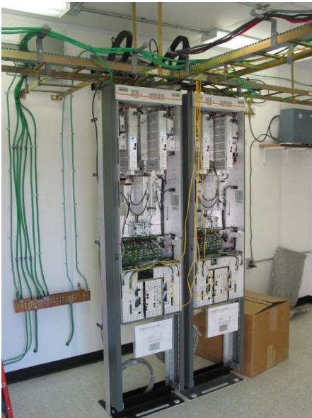
One of many switch and equipment cabinets at Dominion
